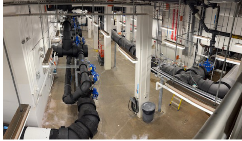
Water Treatment Plant Pipe Gallery
