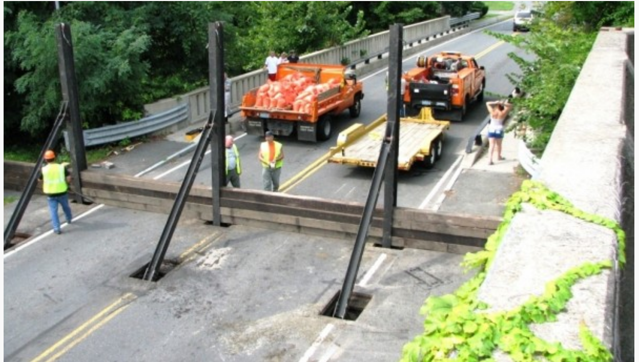
On Saturday morning, DPW workers were busy installing floodgates to stop the Mill River from flooding downtown. (David Reid photos)
