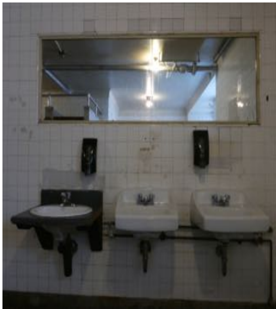
Men's restroom mirror mounted high
