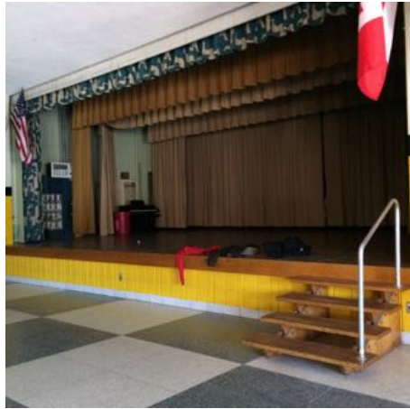
Stairs have non-compliant handrail and open risers, no access by ramp or lift
