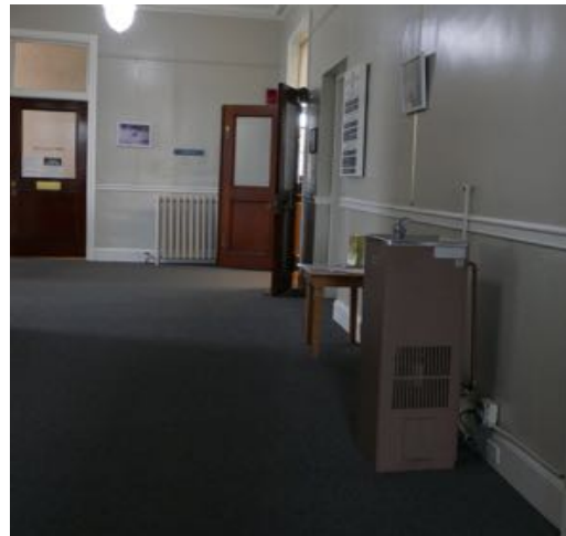
No low drinking fountain in building
