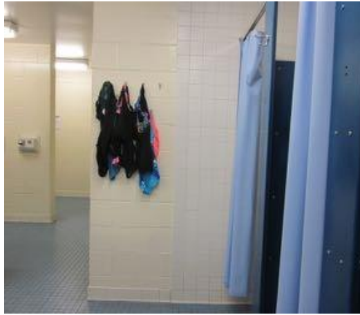
No hook within reach of accessible stalls in locker rooms
