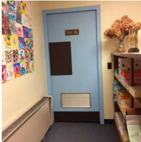
Sign at 2 nd floor toilet rooms indicates accessible, but non-compliant sign on door
