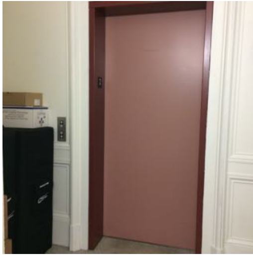
Furnishings impede clear floor space at elevator
