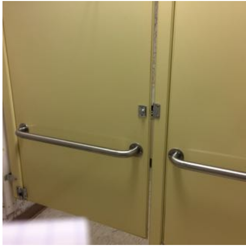
Door swings into stall, grab bars non-compliant
