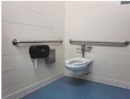
Inside flush at women's locker room stall
