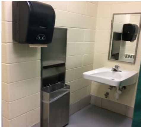
Paper towel dispenser protrudes and is above maximum reach range
