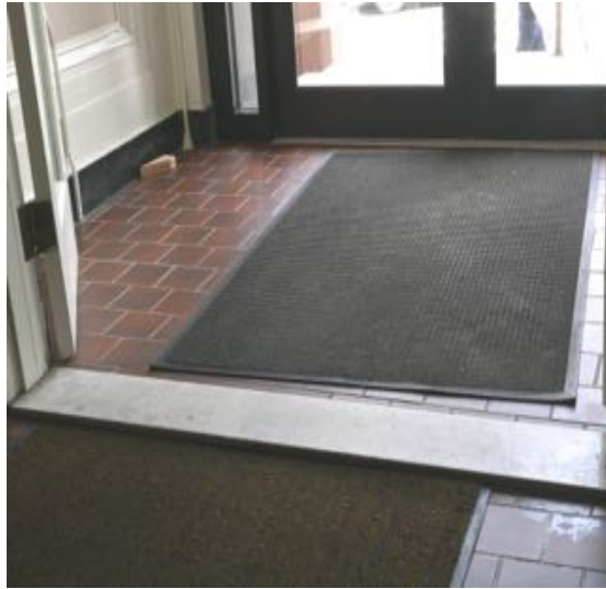
Trip hazard at front entry threshold
