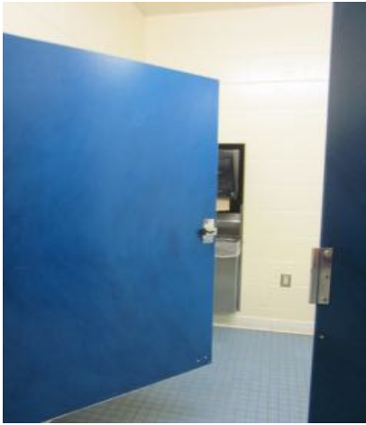
No pull hardware on either side of stall doors in locker rooms
