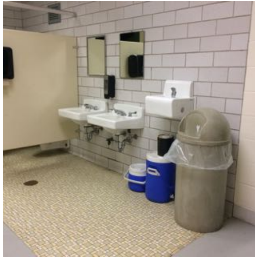
Sinks, dispensers, mirrors non-compliant at Girls' locker room
