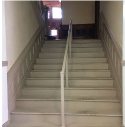
Handrails on stairs not compliant
