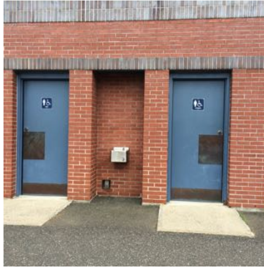
Outside toilet rooms: doors heavy, drinking fountain non-compliant; signage mounted on doors
