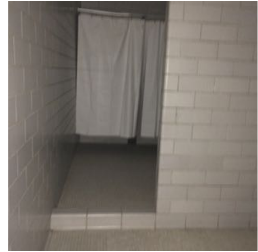
Non-compliant showers at Girls' locker room
